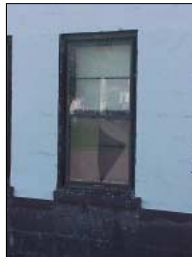
Figure C-15. Exterior window pane is broken, but interior window paint is intact.
