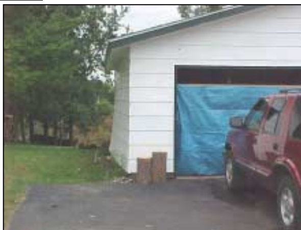
Figure R-11. Garage door failure led to deformation of garage wall. (800 Menasha Avenue, Ladysmith)
