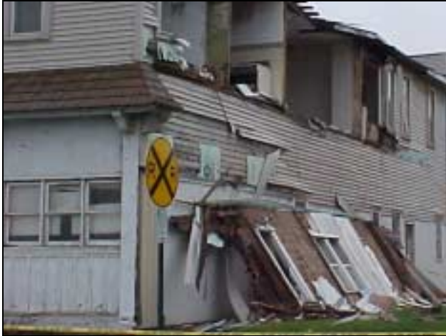
Figure C-21. Second floor wood framing failure. (Minor Ave. Ladysmith)
