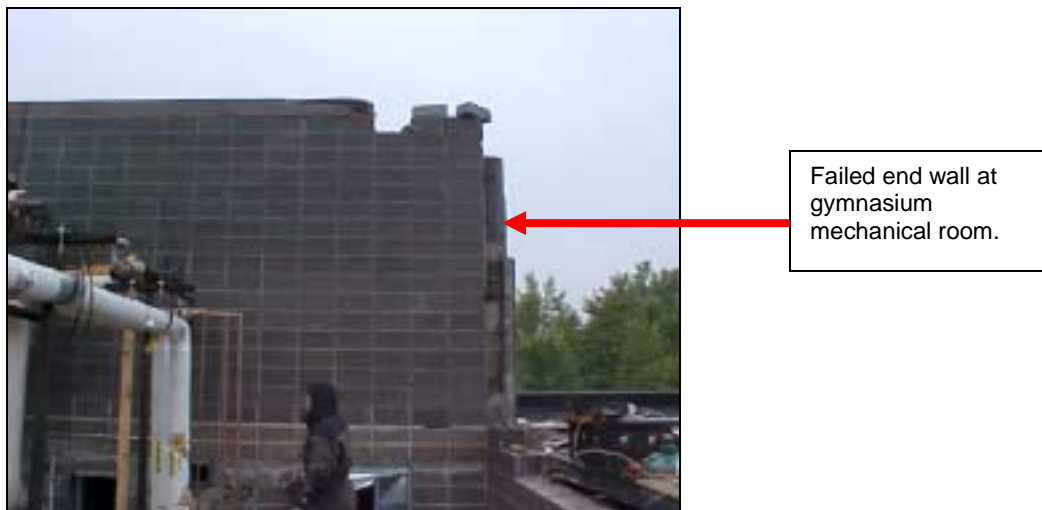
Figure S-7. The non-load bearing endwall in the mechanical room (missing from right side of photo) at the gymnasium failed from lateral wind pressures and instability at the top of the wall caused by the failed roof decking.
