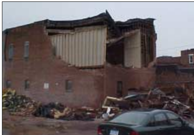
Figure C-7. Failure of 2 nd story brick masonry walls from lateral wind forces.
