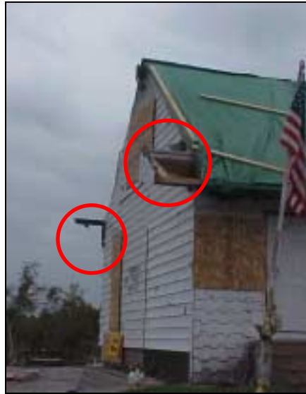
Figure R-6. Large overhang roof failure. (307 Lake Avenue, Ladysmith)
