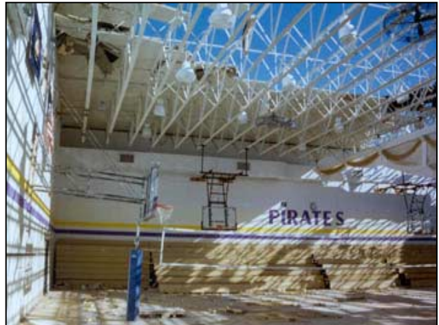
Figure C-11. Tectum roof deck loss at the Gilman School (Courtesy of the Gilman School).
