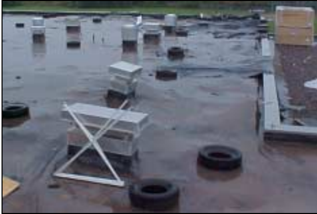
Figure C-9. Uneven roof decking and roof insulation and displaced roof vents above classrooms.
