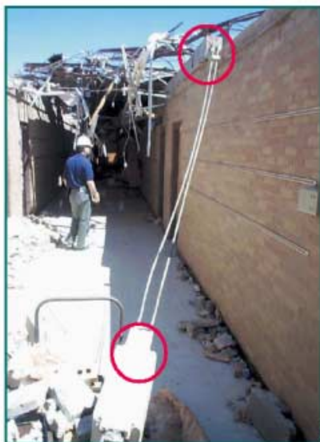
Figure C-24. Bond beam detached from top of CMU wall (with brick veneer). There was no connection between the bond beam and the top of the wall. (From FEMA 342).
