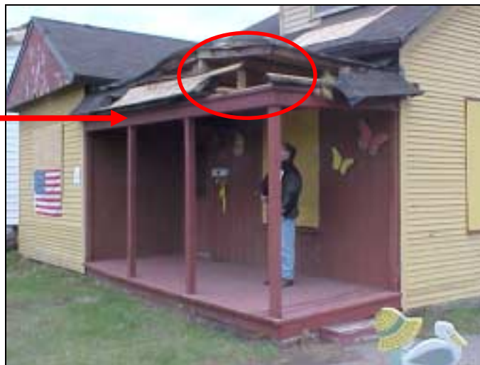
Figure R-5. Damage to overhanging porch roof. (421 Lake Avenue, Ladysmith)
