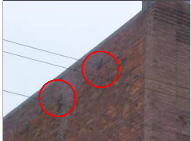
Figure C-27. Brick masonry wall reinforcing on upper story of building (Minor Avenue, Ladysmith)
