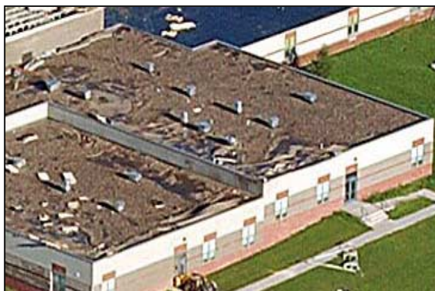
Figure C-8. Roof ballast is missing along roof edges.
