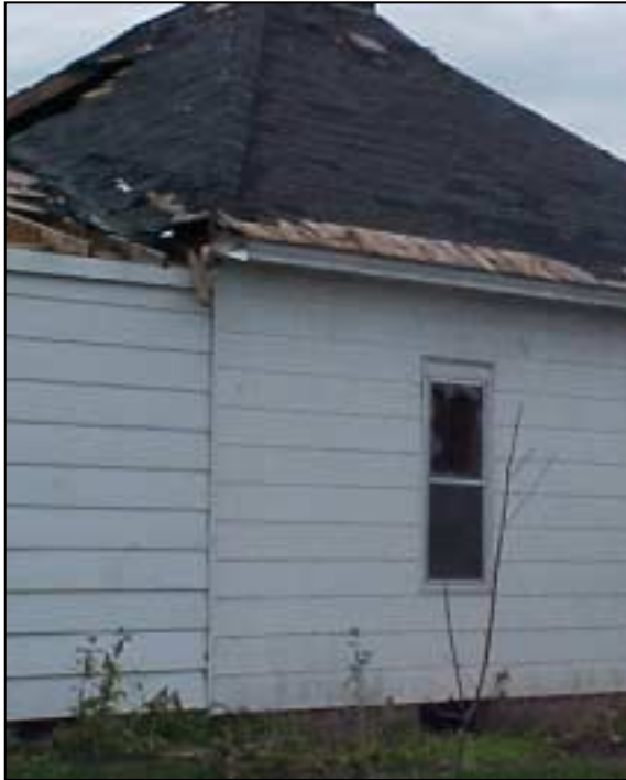
Figure R-19. Typical roof covering damage along roof edge. (507 Lake Avenue, Ladysmith)
