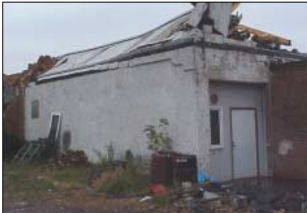
Figure C-3. Second story masonry wall failure. Wall failed from lateral wind pressure probably after roof was separated from structure.
