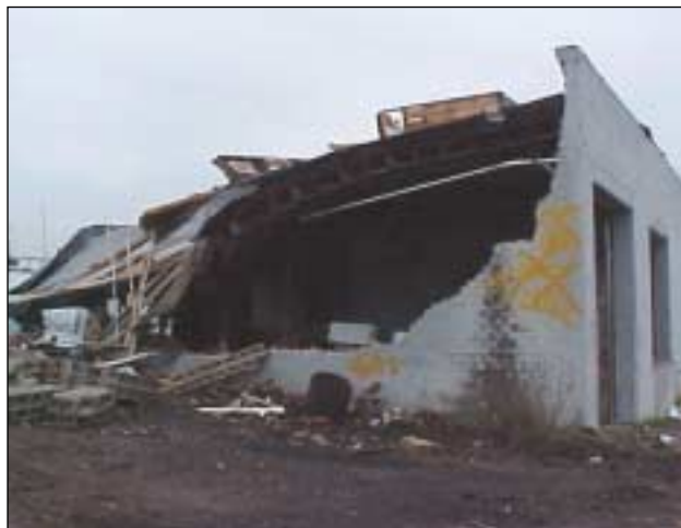
Figure C-5. First floor masonry wall failure. Wall failed from lateral wind pressure probably garage door failed.
