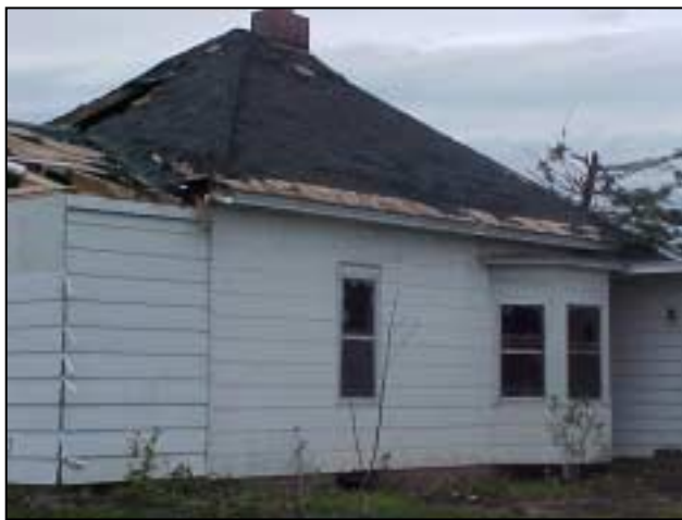
Figure R-2. Loss of roof shingles beginning at roof edge. (507 Lake Avenue, Ladysmith)
