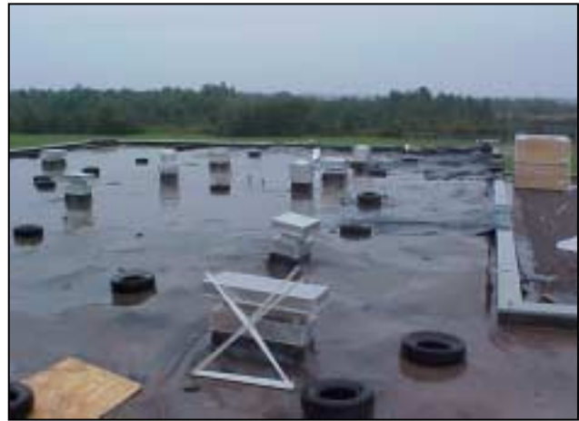
Figure S-4. Roof decking is uneven, insulation boards are uneven under roof membrane, and vents/fan cowlings are damaged. (Note: Gravel ballast was removed so repairs could be preformed.)
