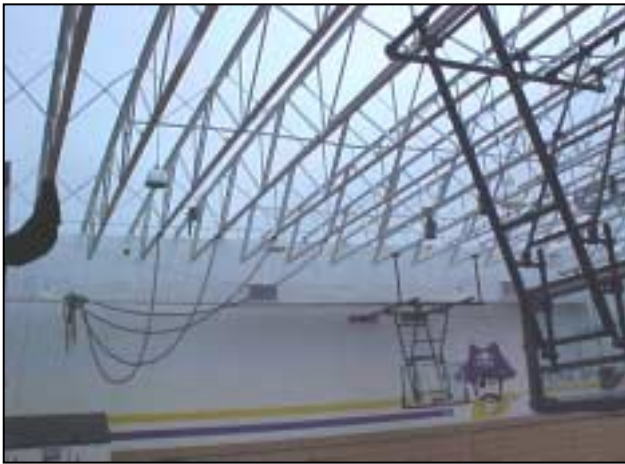
Figures S-3. Missing roof decking in the gymnasium. It should be noted that these walls did not collapse.
