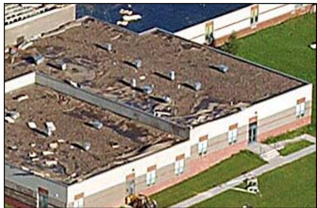
Figures S-2. Damaged roof at Gilman School. Ballast is missing along edge sections of the roof where wind forces are the highest.
