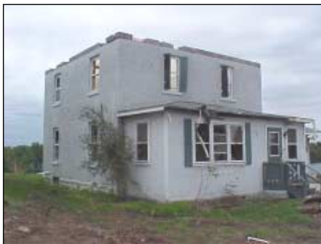
Figure R-10. Masonry house with missing wood roof due to poor connections. (607 Lake Avenue, Ladysmith)
