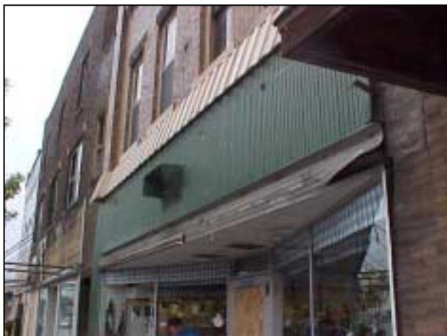
Figures C-30. Awning damage in foreground and intact awning framing in background.
