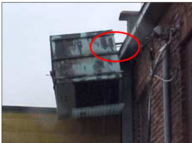
Figure C-19. Roof top unit removed from roof by wind forces. Electrical conduit is all that has kept this unit from falling completely off the roof.
