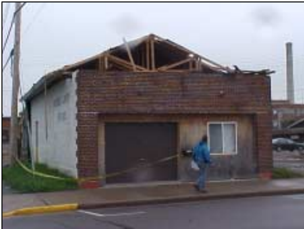
Figure C-10. Gable end wood roof with decking failure. Loss of decking may have lead to instability and failure of end trusses.
