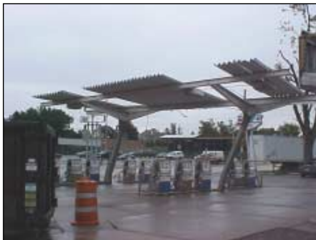
Figure C-31.. This gas station canopy can be replaced with a new canopy designed to resist high winds.
