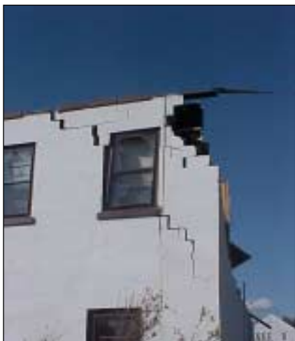
Figure C-4. Second story masonry wall damage. Uplift on roof caused step cracking in wall.
