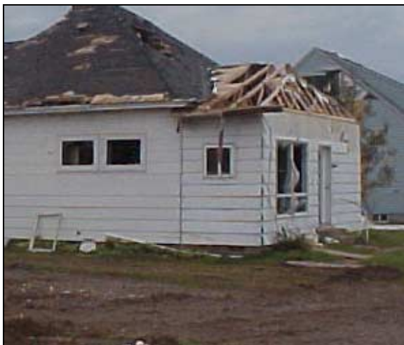
Figure R-7. Hip roof success, gable end roof failure
