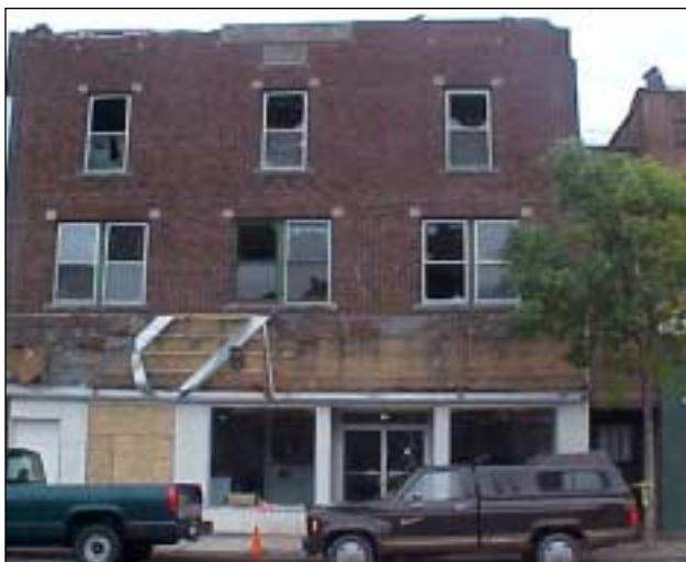
Figures C-14. Typical window damage to commercial buildings.
