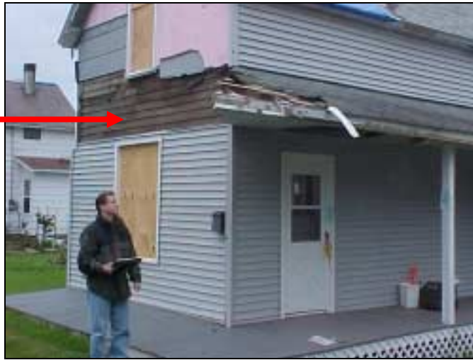
Figure R-4. Failure of overhanging porch roof. (923? Lake Avenue, Ladysmith)
