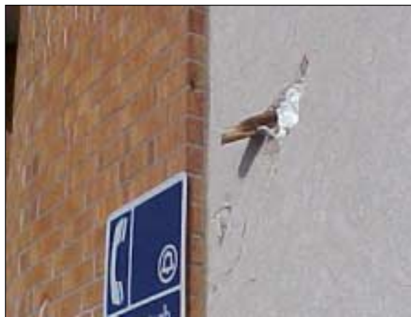
Figure C-17. Windborne debris impacted into EIFS wall system.
