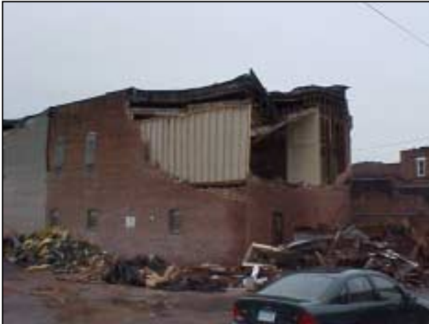
Figure C-26. Typical second story brick masonry failure. (between xx Avenues, Ladysmith)
