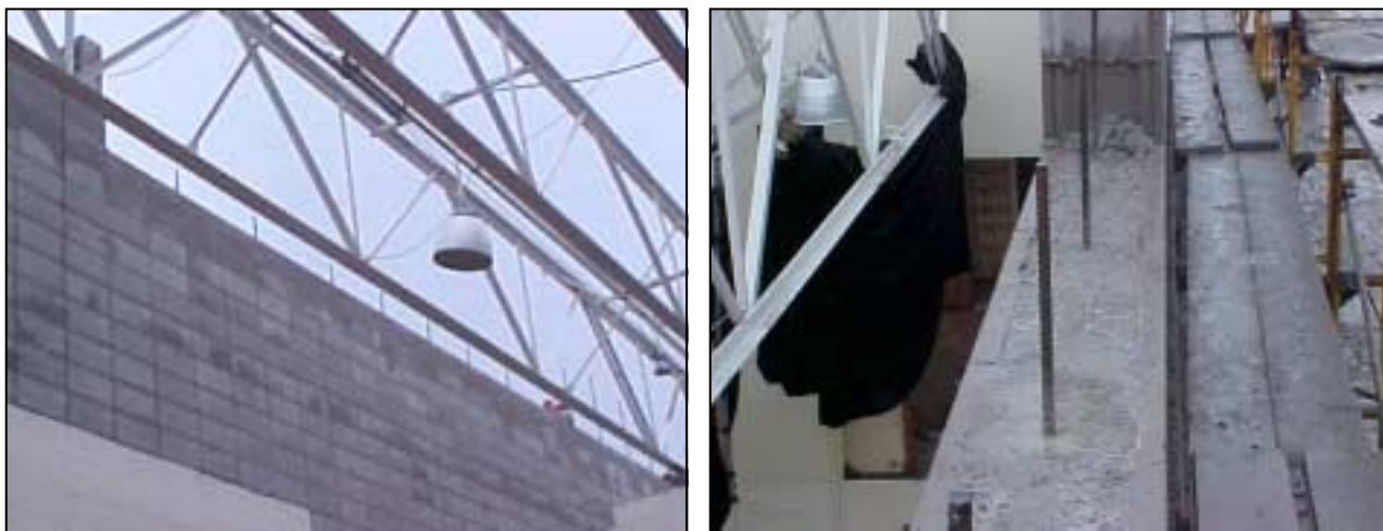
Figures S-8 and S-9. Vertical reinforcing steel being installed in the gymnasium endwalls. The reinforcing steel spans the length of the wall (vertically) and is placed in grout filled cell every 3'-0”.
