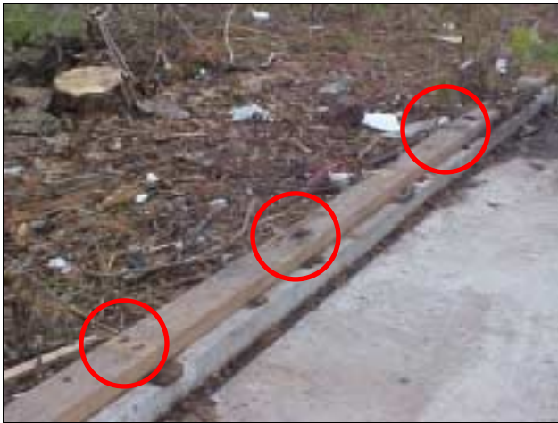
Figure R-18. Failed wall connection to sill plate at a detached garage. Toe nail marks from wall studs are circled. (415 Lake Avenue detached garage, Ladysmith)
