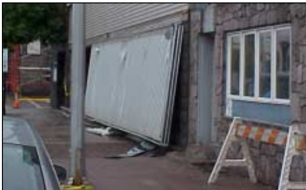
Figure C-18. Damaged store awning. The cantilevered awning failed from wind uplift forces.
