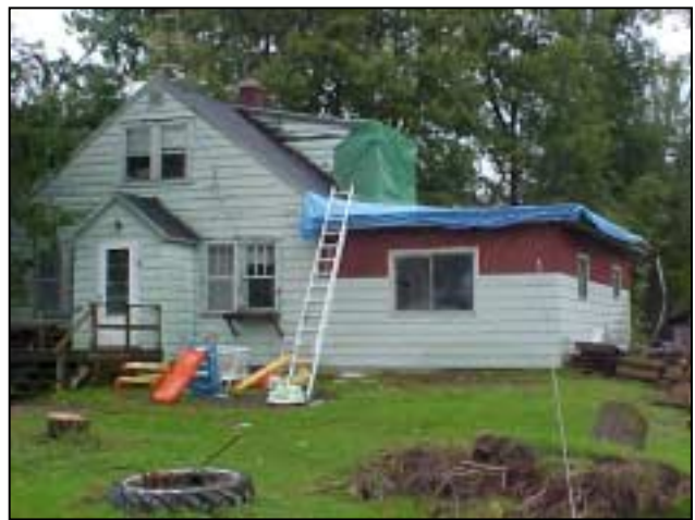
Figure R-3. Loss of roof shingles and sheathing. (unknown address, Gilman)
