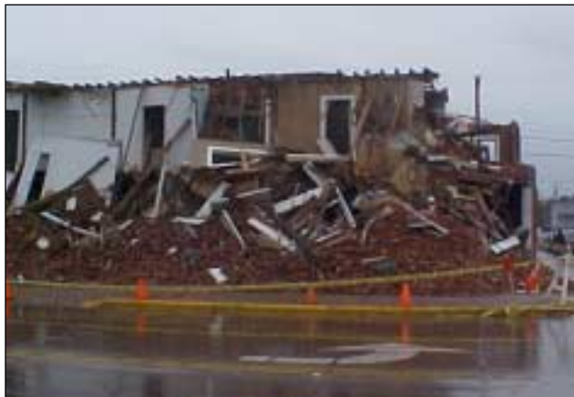
Figure C-6. Completed failure of 1 st and 2 nd story unreinforced brick masonry walls.
