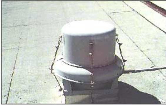
Figure C-32. Example of well-secured roof top unit to resist lateral and uplift wind forces (Source FEMA Archives).
