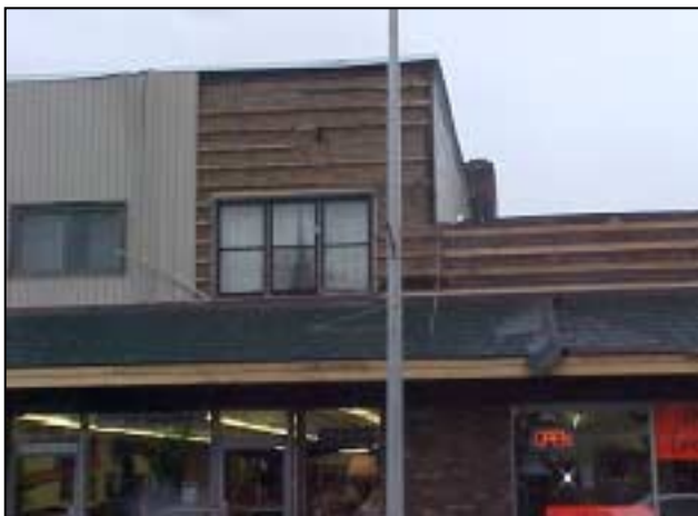
Figure C-16. Siding damage from wind suction forces.
