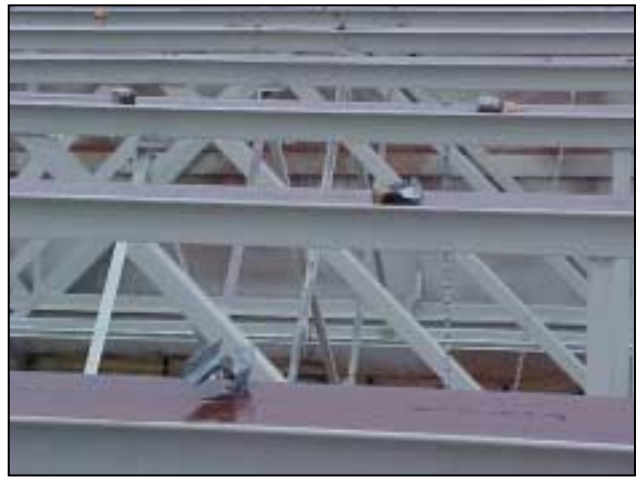
Figure S-6. Clips from the tectum roof deck system at the gymnasium. The loss of the roof deck was a result of the inability of these clips to restrain the deck or the failure of the deck itself at the clips.
