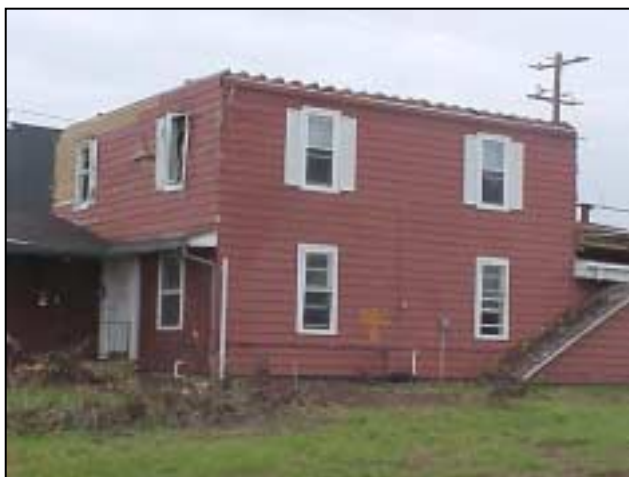
Figure R-9. Wood-frame house with missing wood roof due to poor connection at top of wall. (Multi-family house on Lake Avenue, Ladysmith)
